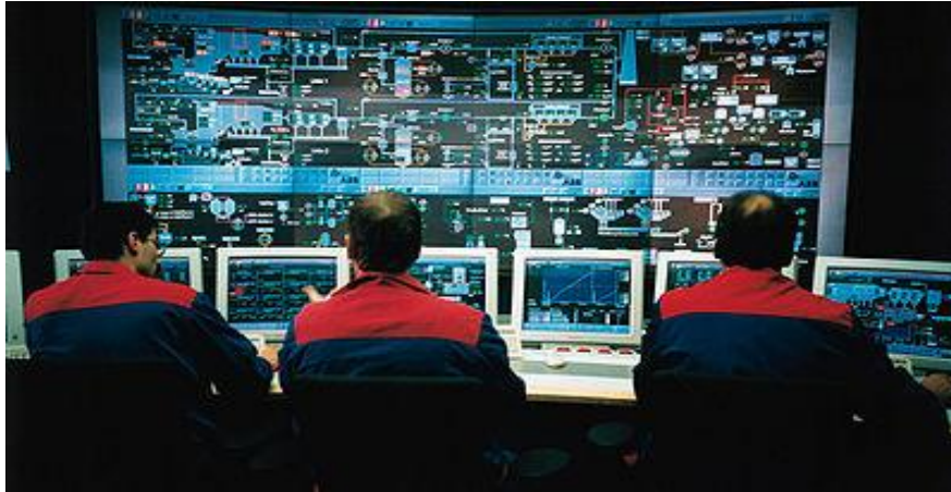
Figure 2.1: WTE Control room of a typical moving grate incinerator overseeing two boiler lines Sources: Themelis, Nickolas, (2003).
